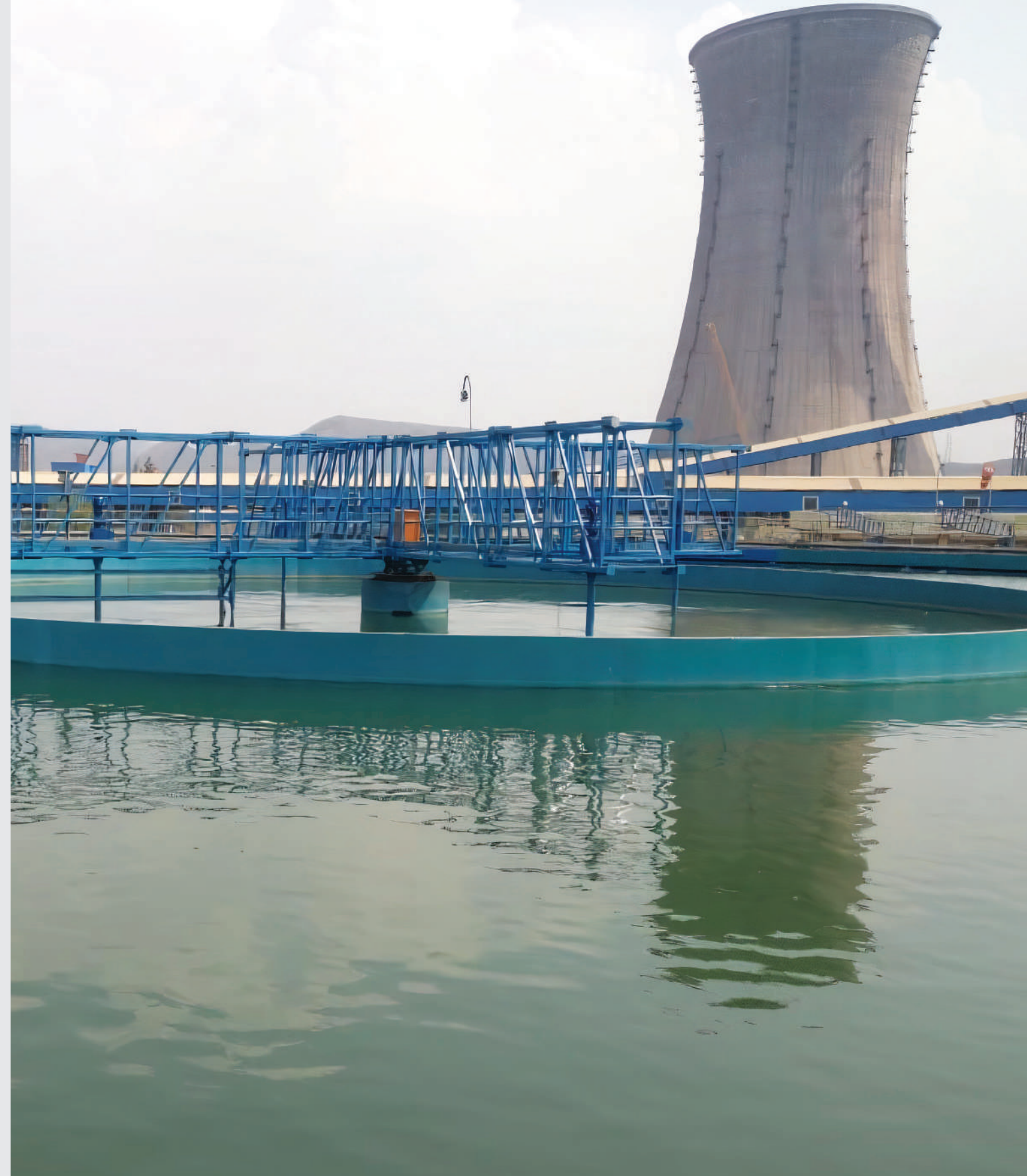
▲ Water treatment and management project at Karnataka Power Corporation (KPCL) site
