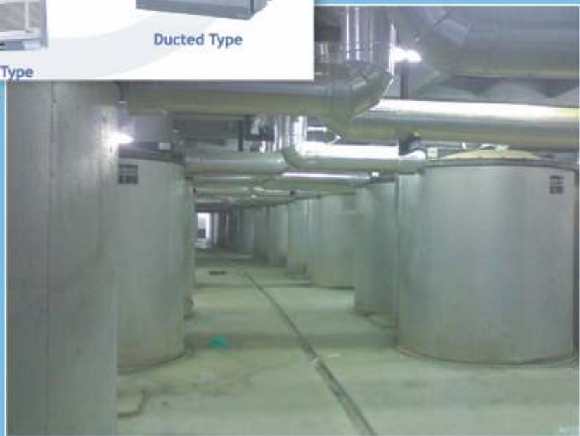
Thermal energy storage system for energy conservation
