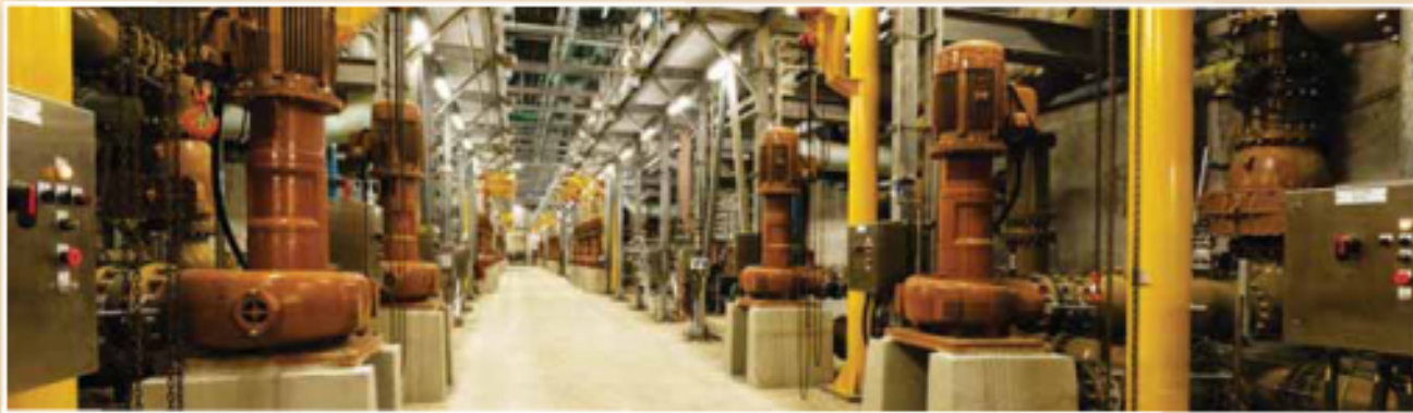
One of the world's largest of its kind. Process equipment and stainless-steel piping for 400 million litres/day.
