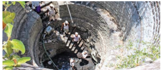
Constructed poly farm ponds and trained farmers on how to increase water availability to resolve the acute water shortage in Dadra.
