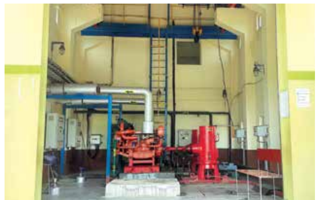
|||||| Gulguli Pumping Station, Cuttack, Odisha
